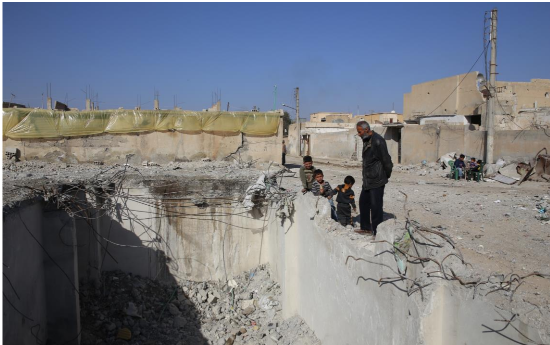
Mohammed Aswad looking down into the basement of his family's building, where his brother and seven other civilians, were killed in a Coalition strike on 28 June 2017. The building was completely destroyed. © Amnesty International
